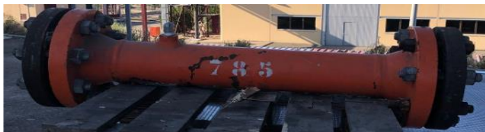
Flange on spool (DN100, PN100). Damaged gasket.
