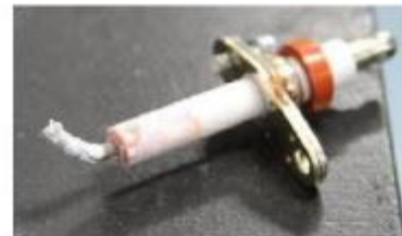
Figure 26: Ionization probe from boiler 1 covered with silica.
